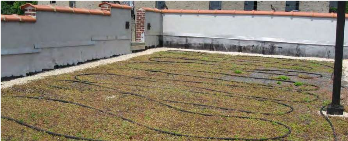
Figure 4-19: Drip irrigation on a constructed green roof at Fordham Bedford Housing in the Bronx.
