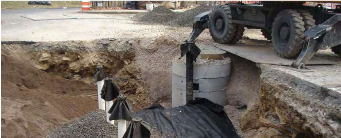
Figure 3-9: Observation wells allow property owners to observe water levels and flush the subsurface system should it become clogged.
