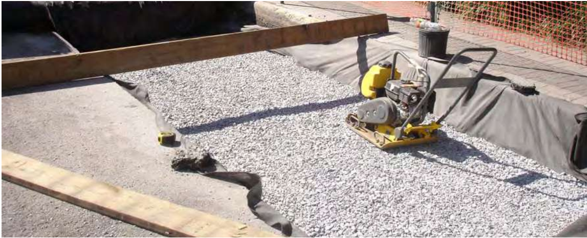
Figure 3-14: Mechanical tampers were used to install the gravel bed below permeable pavers at DPR's Olmsted Center in Queens.
