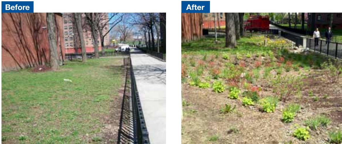
Figure 1-3: Pre and post-installation photos of open space converted to rain gardens at NYCHA's Bronx River Houses.
