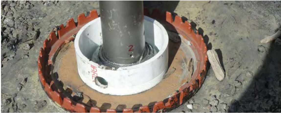
Figure 4-10: The orifice in this controlled flow drain sets the ponding depth and controls the out-flow from the roof on DEP's Storage Facility in Brooklyn.
