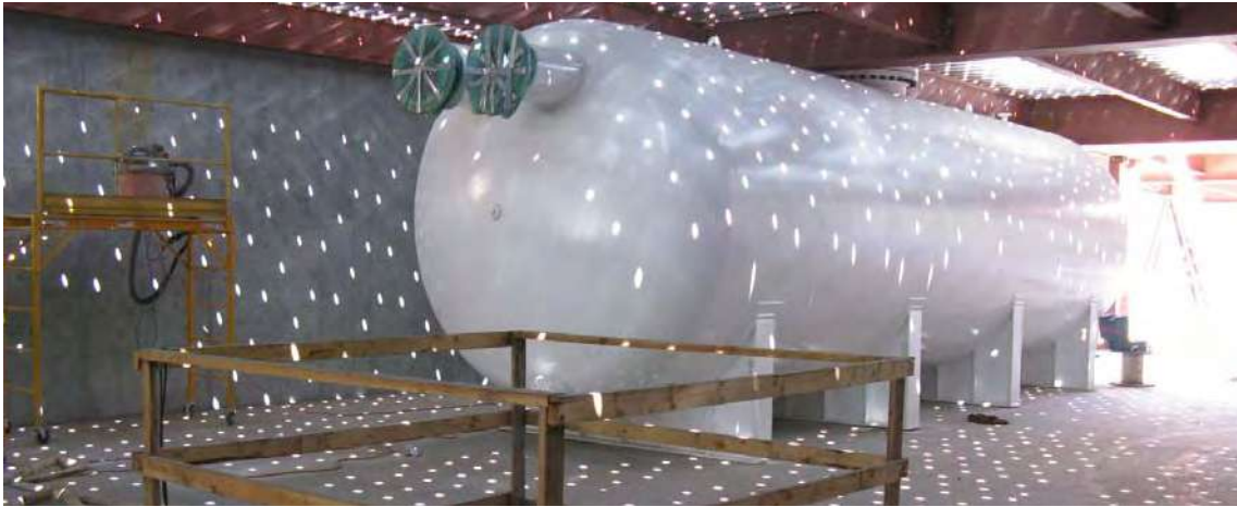
Figure 5-1: A 10,000 gallon tank at Remsen Yard used to store rooftop runoff to wash trucks and settle dust. The site, designed and constructed by DDC, also has a 72,000 gallon retention tank (not pictured), used to collect runoff from the entire site.
