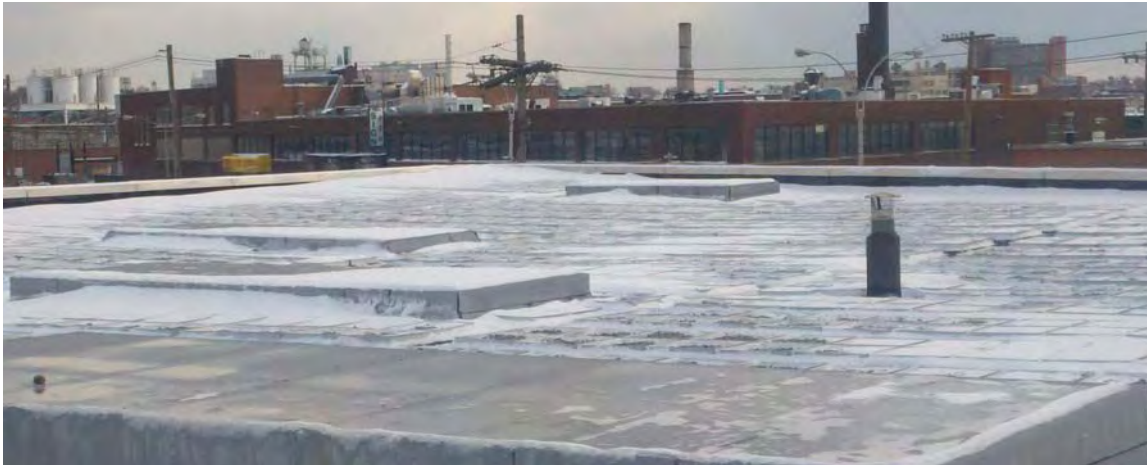
Figure 4-14: Blue roof system during winter installed at DEP's Storage Facility in Brooklyn. Prior to rain events, it may be necessary to clear ice and snow from around roof drains to allow for blue roofs to function properly during the winter.
