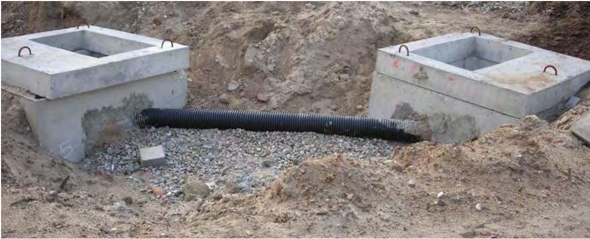
Figure 3-13: Catch basins installed to convey runoff to subsurface systems at Nehemiah Spring Creek Homes at Gateway Estates Phase 2 in Brooklyn.
