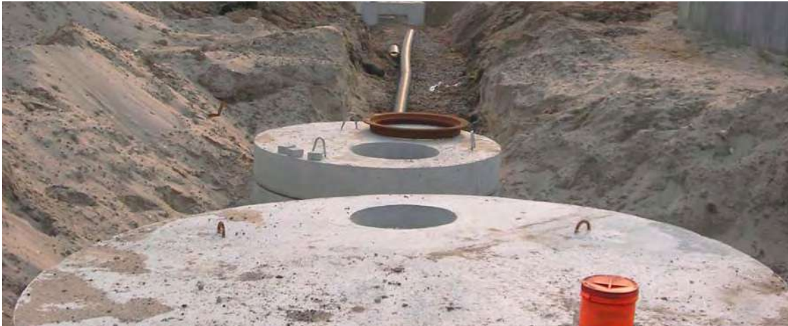
Figure 3-1: Subsurface storage vaults installed at Nehemiah Spring Creek Homes at Gateway Estates Phase 2 in Brooklyn, an affordable housing development sponsored by HPD and the Nehemiah Housing Development Company.
