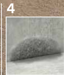
Leaking Areas of Voids i.e. Honeycombing
