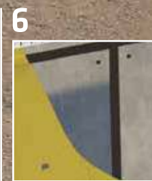
Leaking Compartment Membrane System
