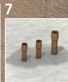
Leaking Penetrations i.e. Pipe Penetrations
